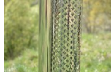
Metal safety fence for heater chimney
