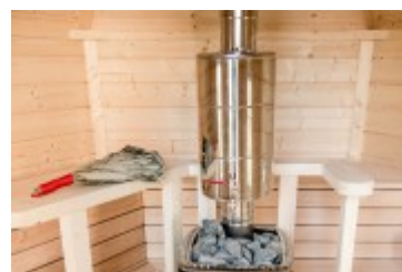
Water Tank For Woodburning Heaters
