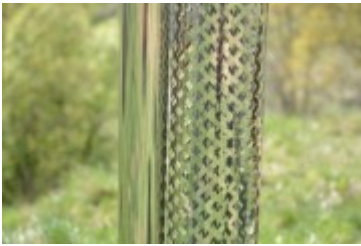
Metal safety fence for heater chimney
