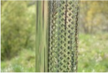
Metal safety fence for heater chimney
