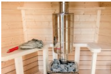
Water Tank For Woodburning Heaters
